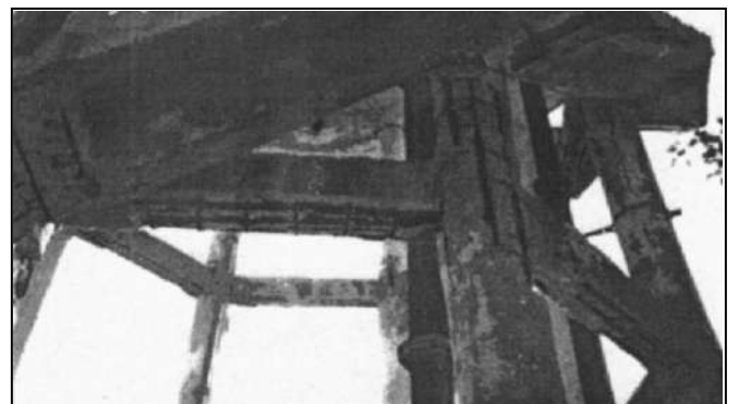
Fig. 6. Corrosion in reinforcement and spalling of concrete in bracings in water tank.
