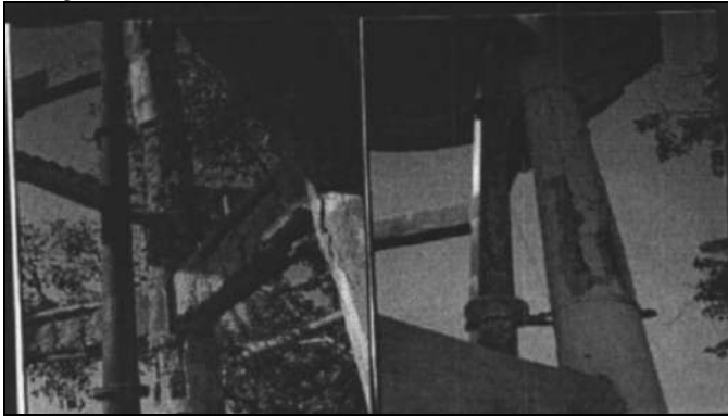
Fig. 11. Vertical cracks and spalling of concrete in columns
