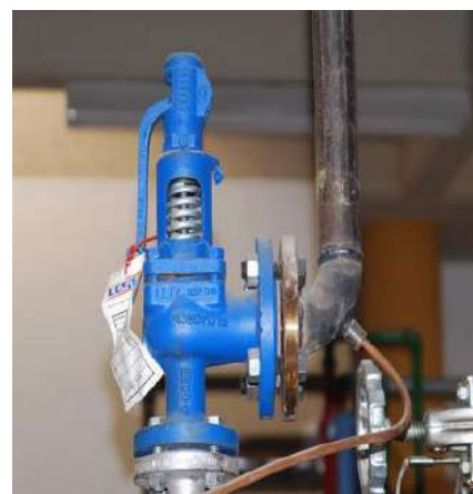
Figure 2 Boiler Safety Valve
