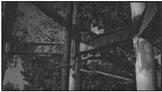
Fig. 10. Spalling of concrete and reduction of reinforcement cross section in bracing, column, and staircase of one water tank
