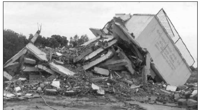
Fig. 3. Collapsed slender and weak framed stagings of water tanks in Manfera village.
